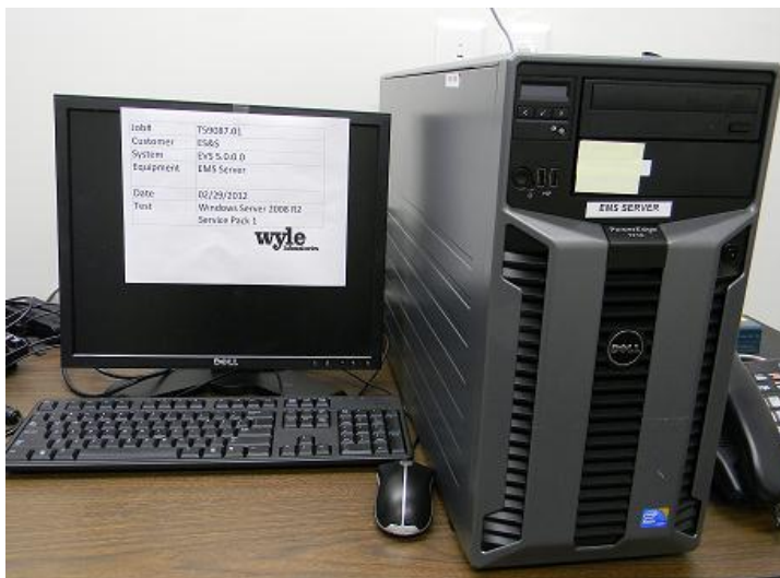
Photograph No. 9: EMS Server
